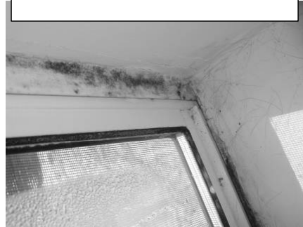
Mold around window where there is no insulation.
