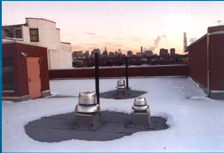
Multi-family exhaust only – new construction
