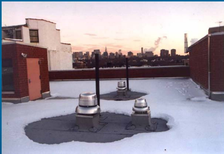
Multi-family exhaust only – new construction
