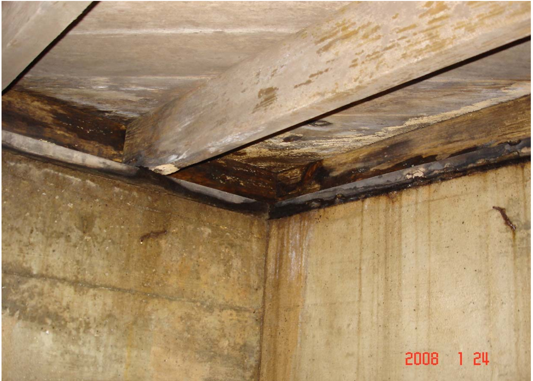
Exercise #2 Moisture & Poor Ventilation
