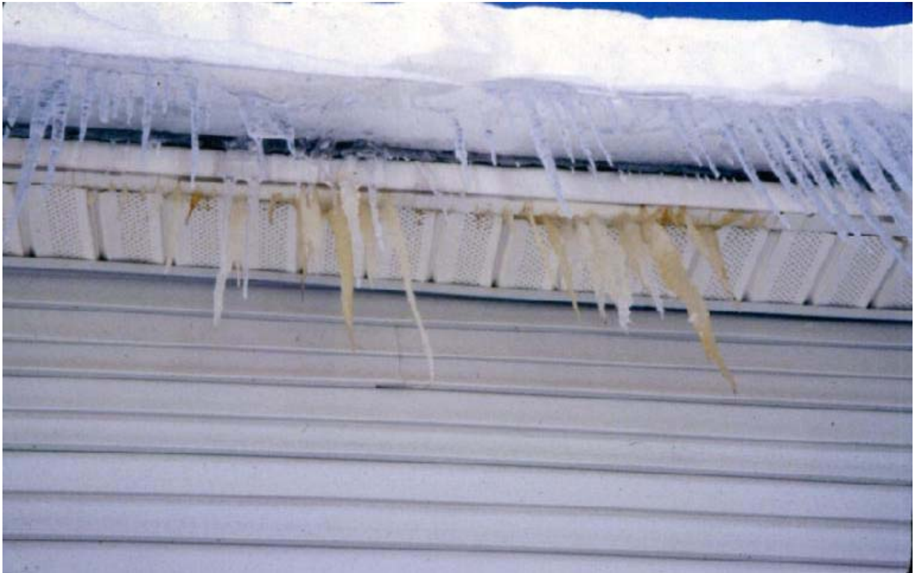
Exercise #2 Moisture & Poor Ventilation
