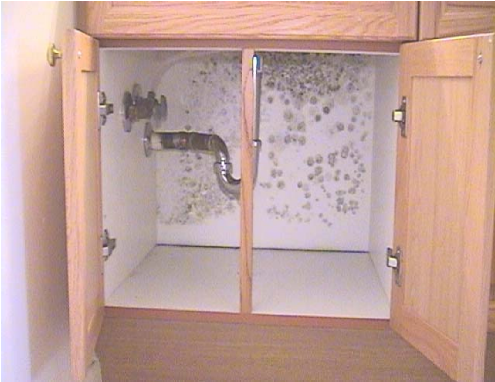
Exercise #2 Moisture & Poor Ventilation
