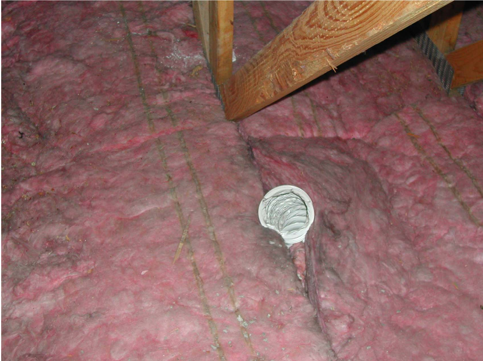
Exercise #2 Moisture & Poor Ventilation
