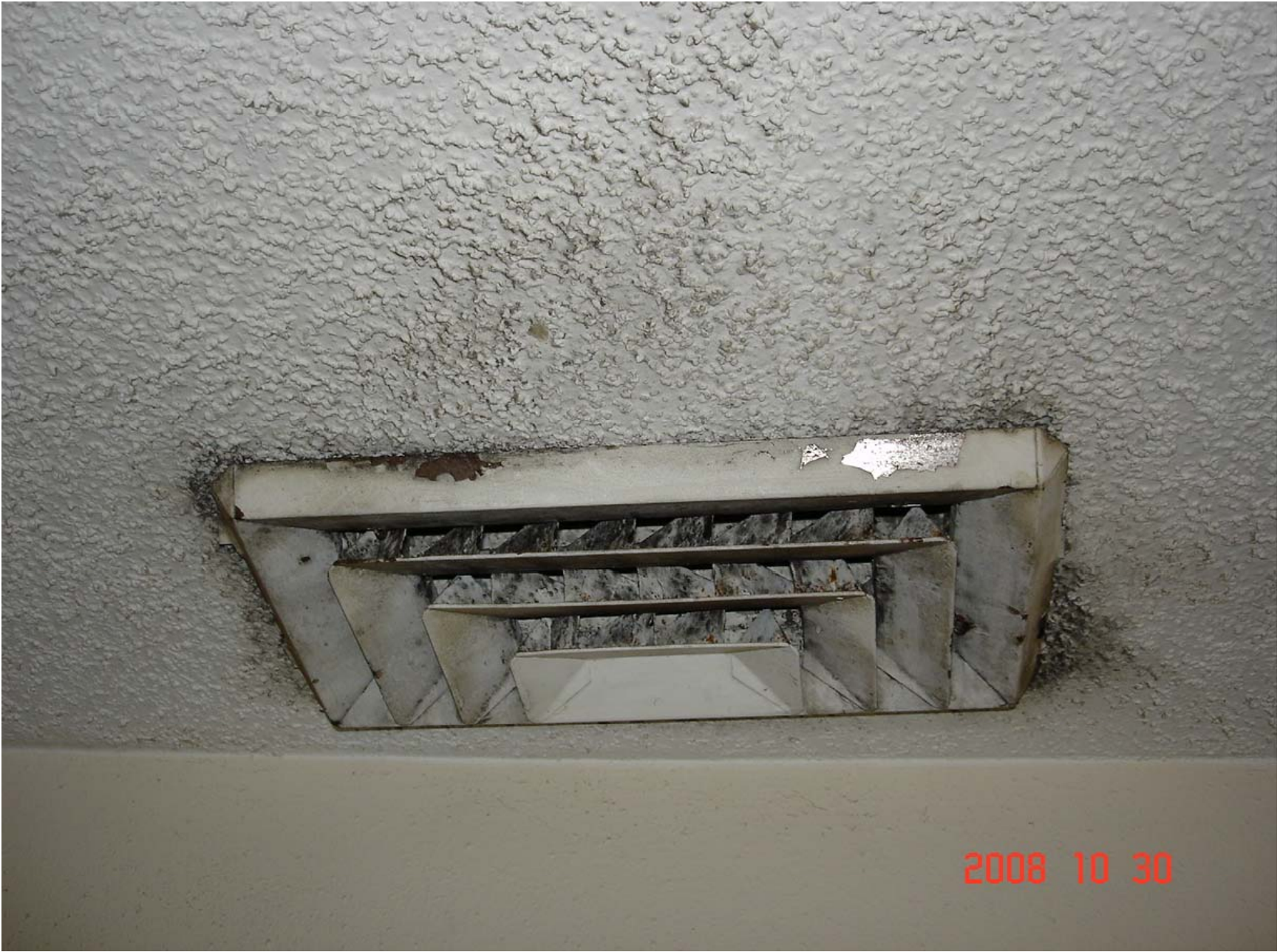
Exercise #2 Moisture & Poor Ventilation
