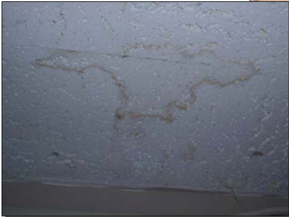
Rodent urine stain in drop ceiling
