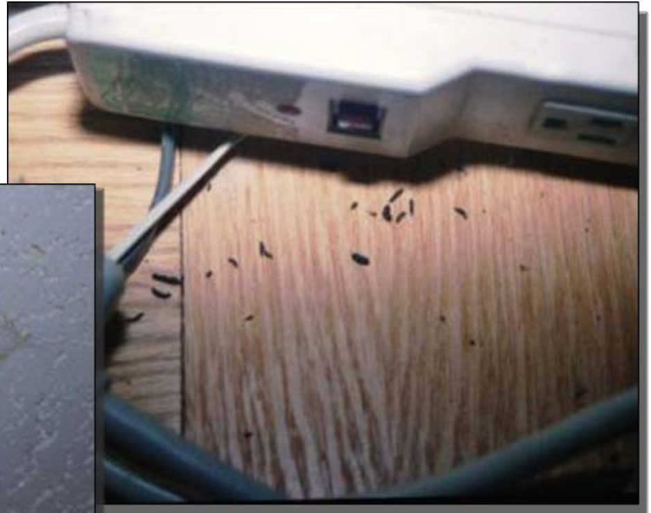
Mouse droppings by a power strip
