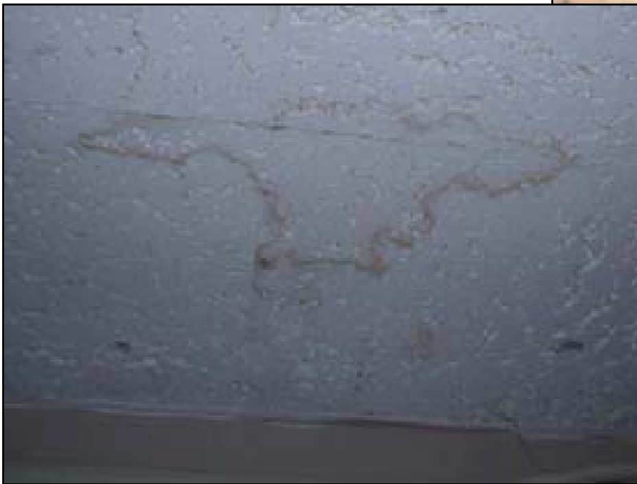
Rodent urine stain in drop ceiling
