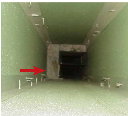
Figure 5 | Leakage point at connection between gypsum board shaft and floor slab (red arrow)
