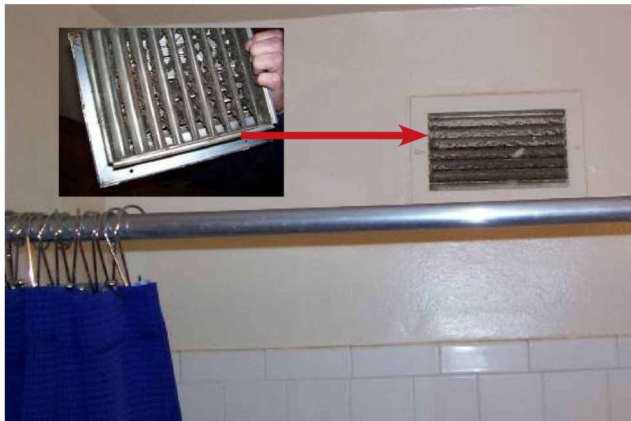
Figure 9 | Dirt and dust clogging grills/registers and restricting airflow
