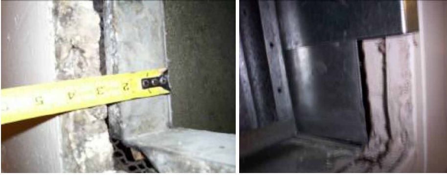
Figure 7 | Leakage between sheetrock and horizontal take-off duct
