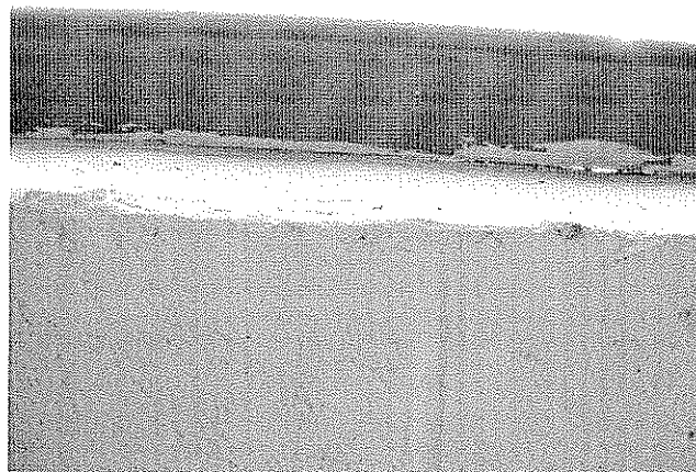
Gap between window frame and opening
