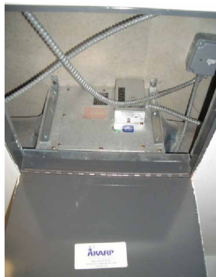
Figure 1 | Inline Exhaust Fan Located above Closet Ceiling
