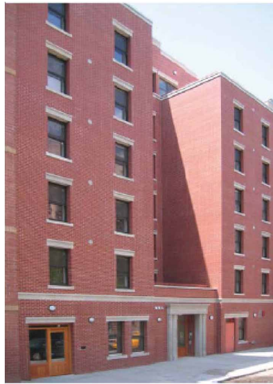
228 E 3rd Street features round metal plates visible on the exterior, which are air louvers for the individual ventilation systems in each apartment.
