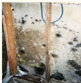
PHOTO 1: Mold and rot from leaving wet insulation in wall.
