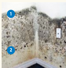
PHOTO 3: Mold growth is heavier in wicking area (above flood level).
