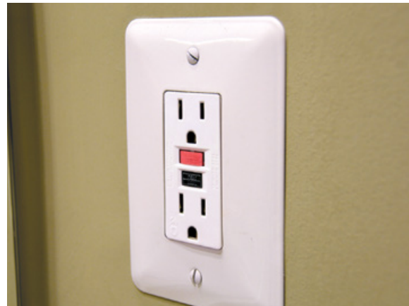
PHOTO: GFCI outlets are safer than other types of outlets in wet areas.
