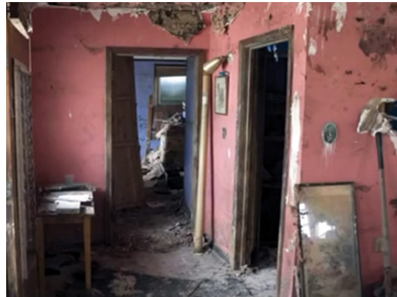
PHOTO: Remain alert to hazardous walking and working conditions.
