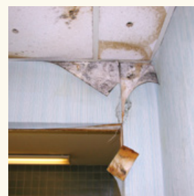
PHOTO 4: Mold behind vinyl wallpaper.
